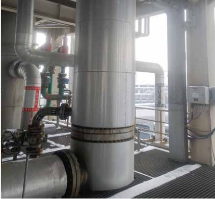
Installation of waste gas TCS heat exchanger in the waste gas recovery workshop
