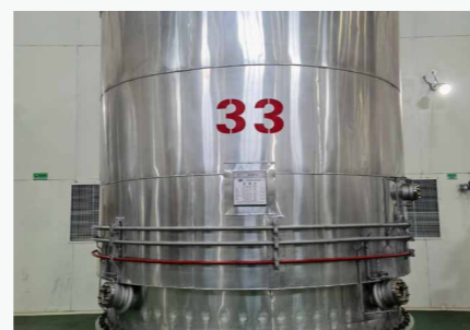
Furnace Power Consumption Reduction and Technical Reform
